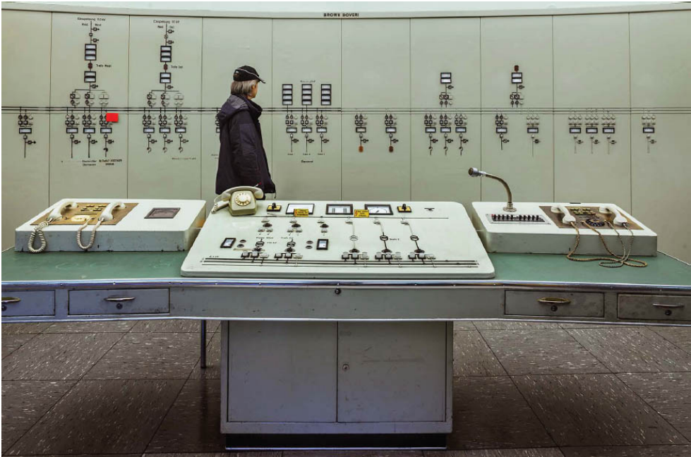
Figure B-1: Switching center (24mm, ISO 100, 1/3 sec., f/9)
